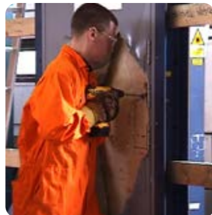
With the door skin removed, a drill is used to attack the hardware.
